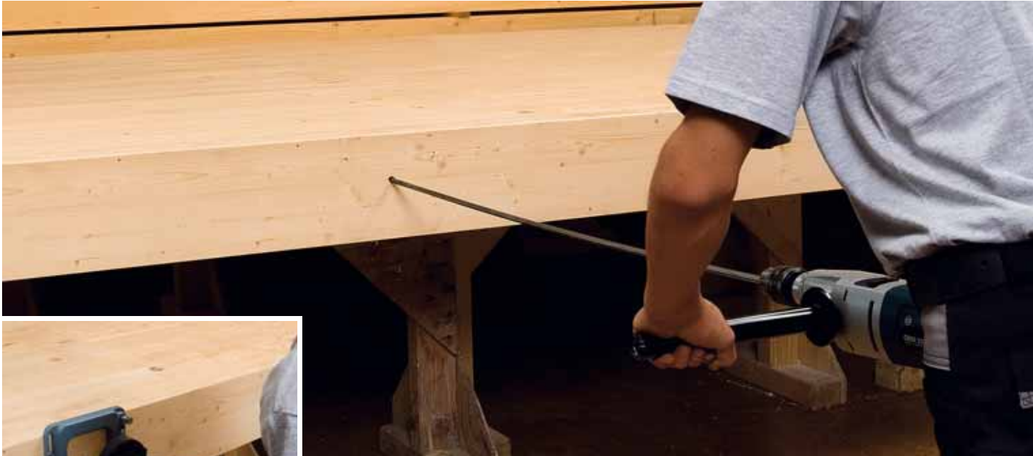
2. Holes up to 3 metres deep can be drilled using the bit extensions of the WB System.
