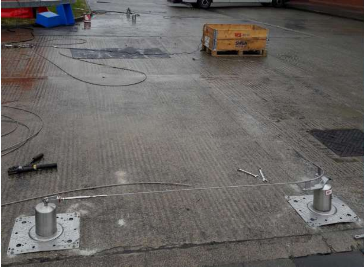
Figure 5 – Horizontal anchor line described as “SOTER II”
